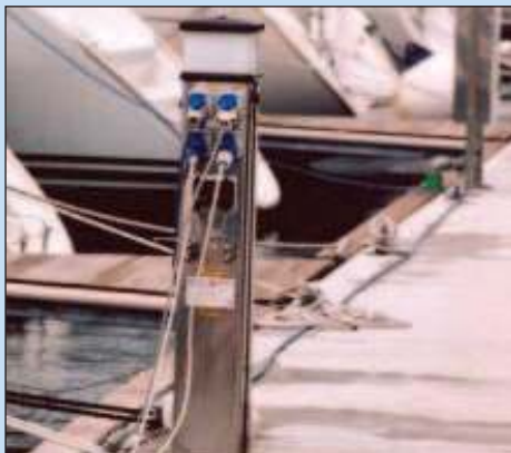
Electrical distribution pedestal
