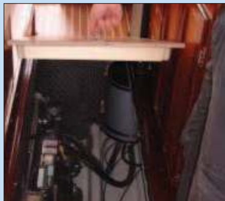
Main engine space
