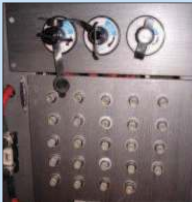
Electric installations on the boat
