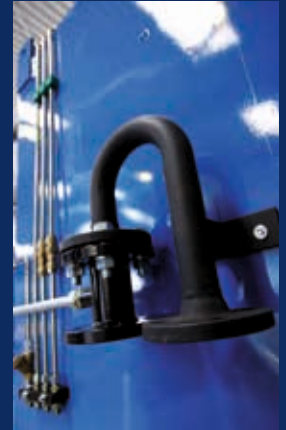
Self-cleaning strainer in the sludge line
