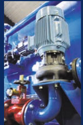
Mill pump ensuring comminution of any solid particles
